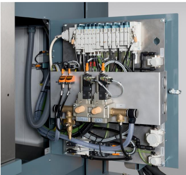
Figure 4: Easily accessible pneumatic control unit
