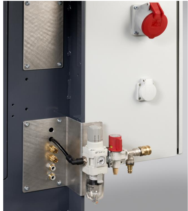
Figure 3: LOTO points, compressed air, cooling water, welding gases, electric power
