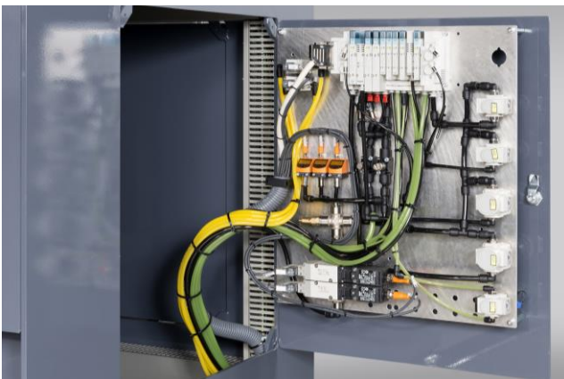
Figure 5: Easily accessible pneumatic valve terminal
