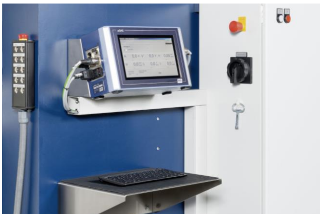
Figure 23: HKS Welding data monitoring system
